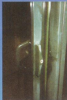
Examples of solvent misuse on a powder coated surface after a 3 year period.
